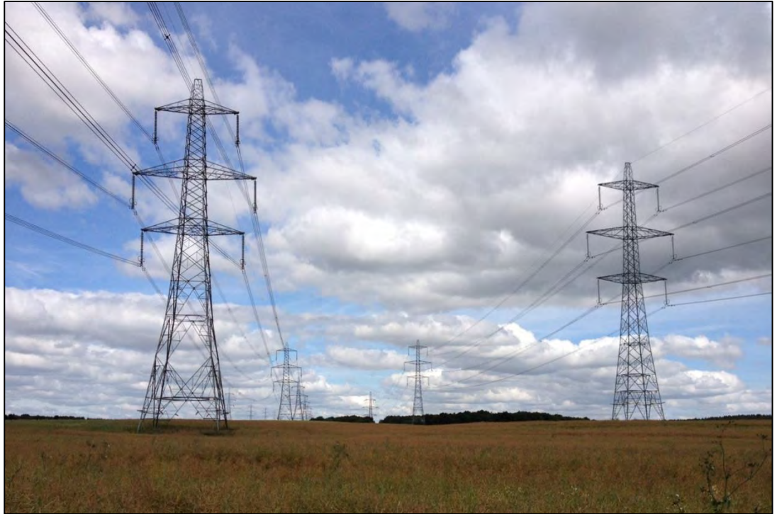
Photo 7.2. Parallel Overhead lines in County Durham with a route transposition to the left in the middle distance.
